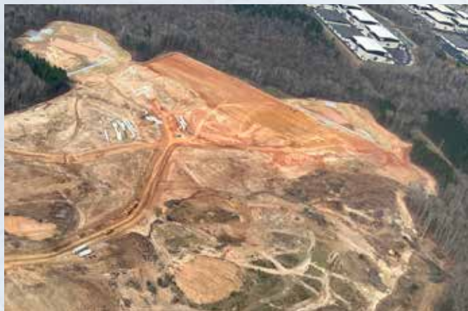
Mass grading of a 600-acre data center development in Fayetteville as seen from above. Georgia's erosion and sedimentation laws are enforced by a mix of local and state inspectors. Georgia's Environmental Protection Division, which is responsible for enforcement in 380 jurisdictions, has about 12 inspectors to cover the state.
